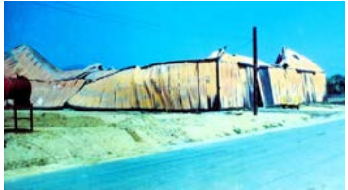
When the sun came out the next morning, damage and destruction were everywhere. This is the charred warehouse I passed in the morning.
